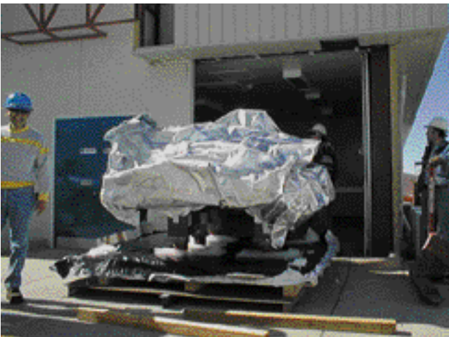
Figure 4: Moving the 2.5-ton Laser Table inside the MMU Laboratory. The wall had to be removed for this purpose.
